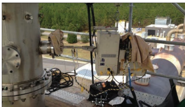
Figure 4: Probe aligned in stack
